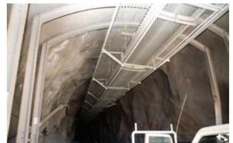
Conveyor entering decline
