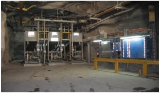
Underground Pump Station
