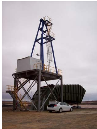
Egress System Installed over Surface Fan
