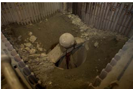
42" Gyratory Crusher and RoQM Bin
