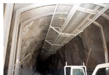
Conveyor entering decline
